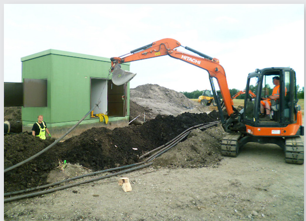
Connection of a transformer station
